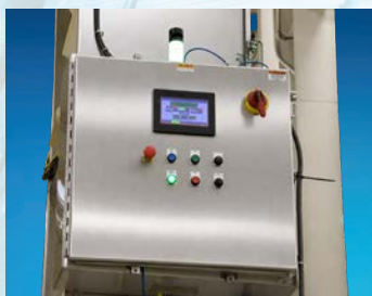
PLC CONTROLS WITH TOUCHSCREEN HMI
